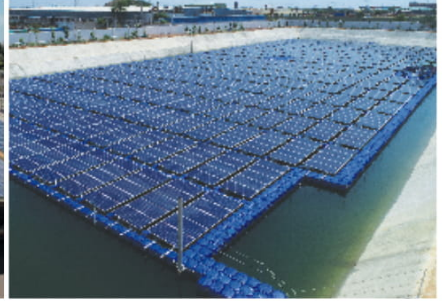
Floating Solar 540 kW, Tata Chemicals, Nellore
