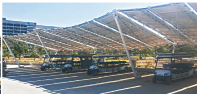
50 kW Solar Vehicle Charging Station at Gujarat Secretariat
