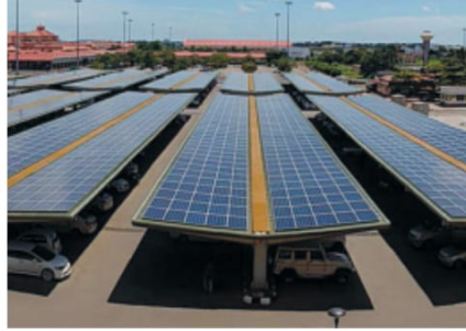
Carport 2.67 MW Cochin International Airport
